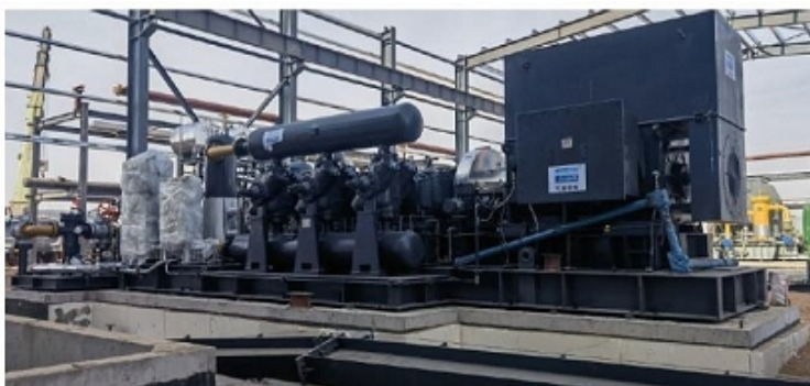
Our ultra-high pressure gas injection compressor unit.
