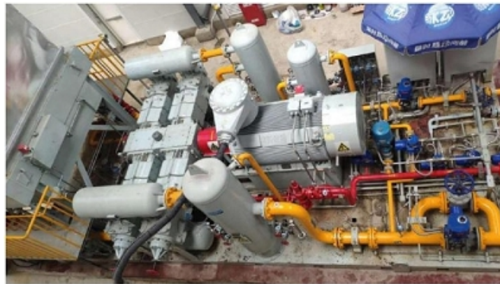
Our gas transmission compressor unit.
