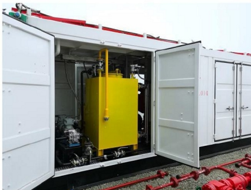
Our Sulphur Removal Device.
